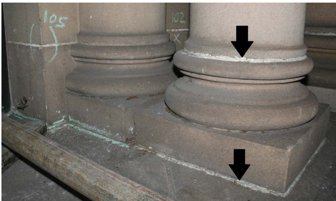
Image 2. Sydney Town Hall: East Facade. The joints indicated by the arrows have been repointed with an off-white putty which laboratory testing showed contained asbestos. The crudeness of its application was one of the dominant visual clues allowing its consistent identification. Laboratory testing showed that the types of pointings evident in all other joints in the image did not contain asbestos. (Image: Peter McKenzie, 4 July 2012)
