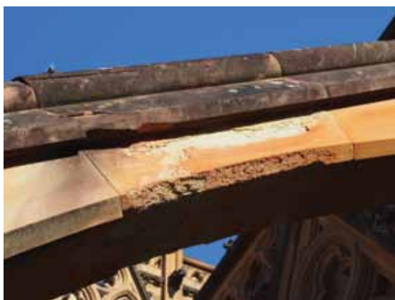
Figure 5. Advanced deterioration necessitates replacement of this stone in a flying buttress.
