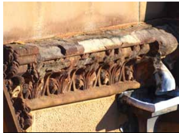
Figure 2. Deterioration of carved cornice cornices in the clerestory.
