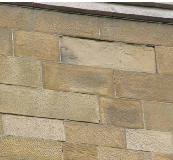
Figure 3. Delamination of face-bedded ashlar, St David's Cathedral, Hobart. (Photo: Jasper Swann, 2008)
