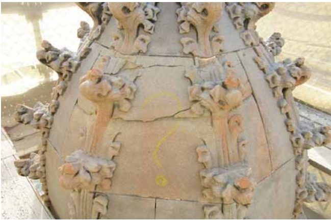
Figure 15. Cracking along a natural plane of weakness. In this instance, the carved stone has sheared through its width completely, and being under little compression, it is at the point where the upper portion of the stone can be dislodged by hand. (Photo: Jasper Swann, 2008).
