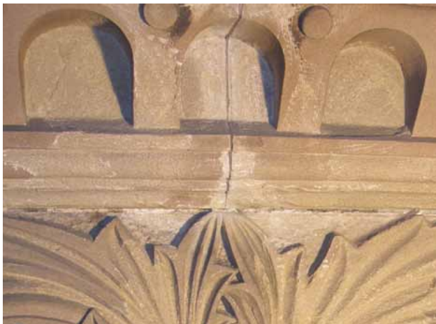
Figure 7. Contour-delamination in the cornice mouldings and carved frieze below, Queen Victoria Building, Sydney, caused by deposition of salts, (visible), beneath case-hardened layer. (Photo: Jasper Swann, 2008)
