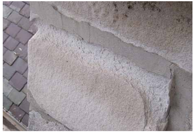
Figure 16. Preferential decay of a buttress stone as a direct result of the unsuitable grey cement mortar used to repoint its upper bed joint. Hunter Baillie Memorial Church, Annandale, NSW. (Photo: Jasper Swann, 2007).
