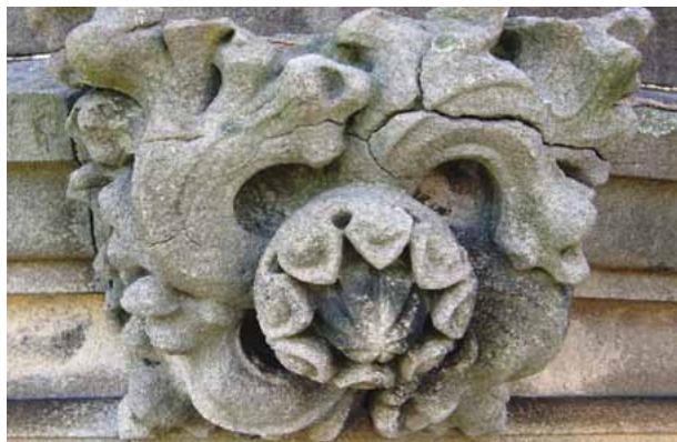
Figure 13. Cracking of a carved boss in Sydney yellowblock. (Photo: Jasper Swann 2008)
