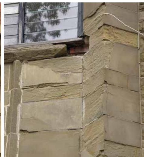
Figure 5. Severe exfoliation of Barrabool sandstone, Newman College, University of Melbourne. (Photo: JS)
