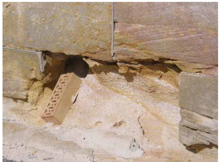
Figure 2. Severe disaggregation caused by salt damp, Spectacle Island, Sydney Harbour. Note the collapse of the vent formerly located in the wall. (Photo: Jasper Swann, 2007)
