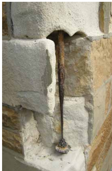
Figure 12. A rusted iron fixing, originally anchoring the spire, has destroyed the quoins on this church tower in Kiama, NSW. (Photo: Jasper Swann, 2009)
