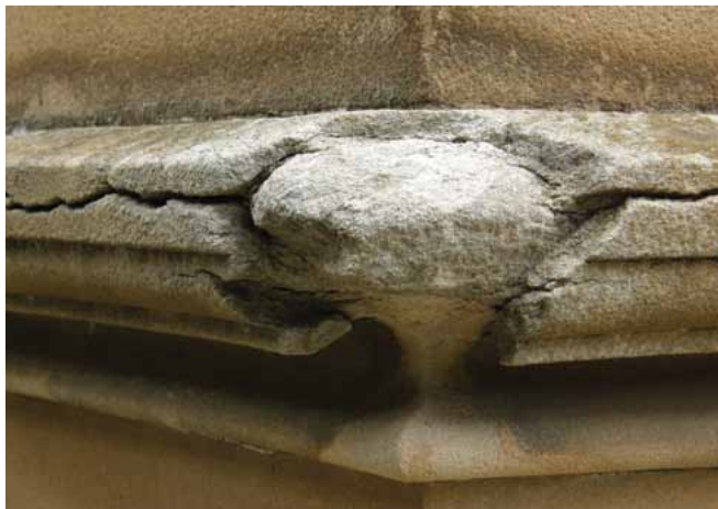
Figure 8. Contour delamination of a Sydney yellowblock string course, Mitchell Building, University of Adelaide. (Photo: Jasper Swann, 2009)
