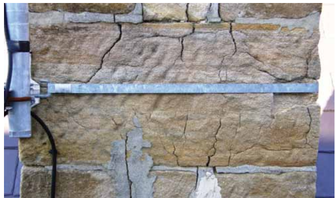
Figure 14. Cracking in a chimney shaft. (Photo: Jasper Swann, 2007)
