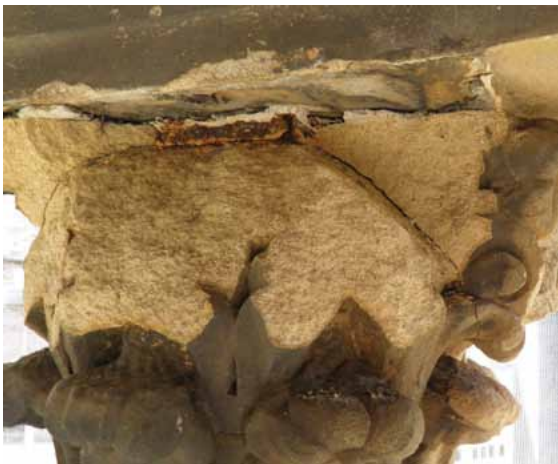
Figure 5. A rusted ferrous plate in the top bed – the cause of significant cracking in the capital.
