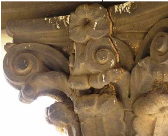
Figure 1. Severe vertical cracking in a capital due to rusting ferrous fixings.
